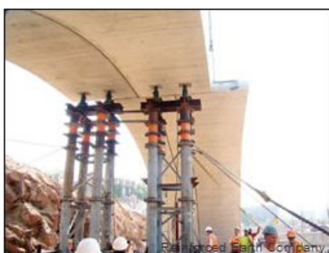
Precast arch segments were lifted into place in a one-step process, requiring one crane.
